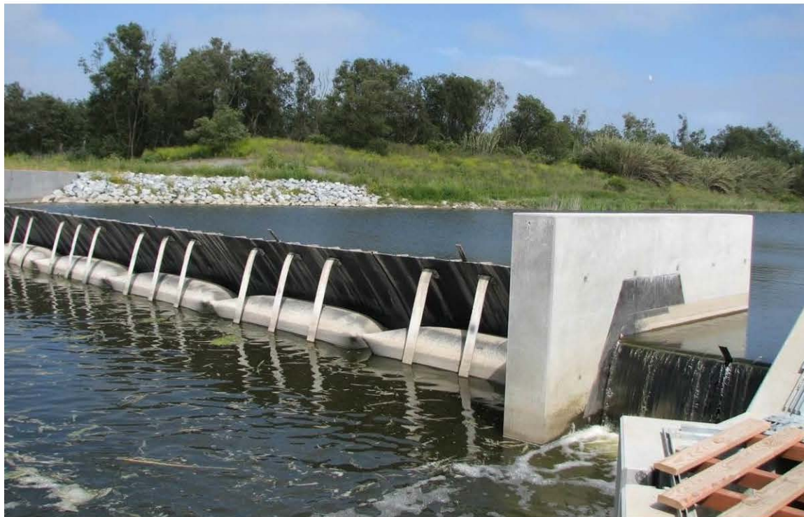
Figure 2.5: SRDF Release Weir
