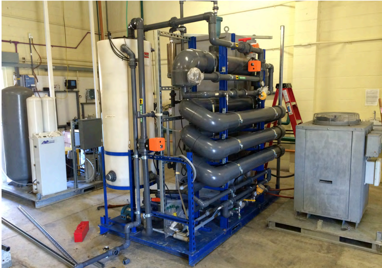
Figure 2.4 - Ozone generation skid (center), chiller skid (right), and oxygen generation skid (back left), during installation
