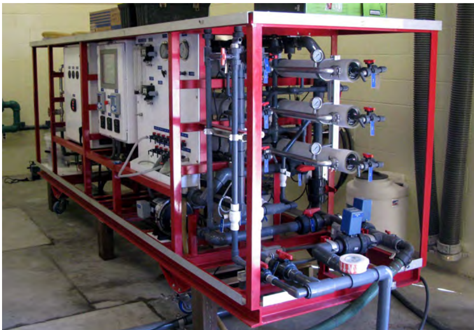
Figure 2.8 - RO Pilot Unit
